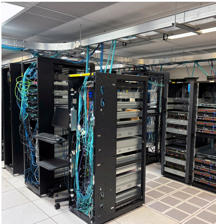
Main Floor - Server Room
