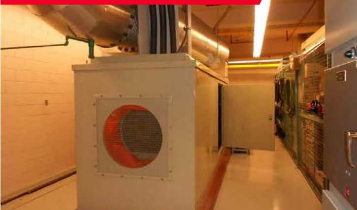
EMERGENCY TURBINE GENERATOR
